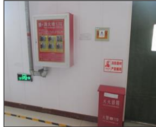
Photo of fire safety equipment Extinguishers and fire hydrant.JPG
