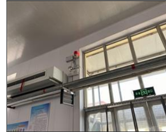
Photo of fire safety equipment Fire alarm testing.JPG
